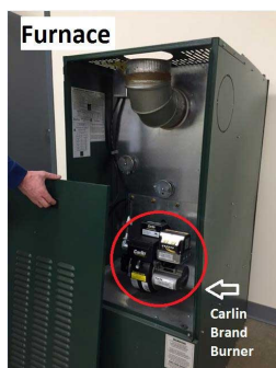
Carlin Brand Burner on Furnace
